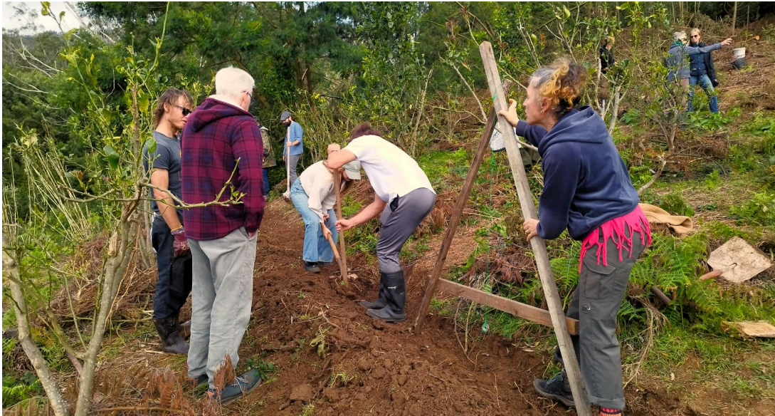
The making of a swale - a level, contour-dug ditch and berm system designed to catch and store rainwater runoff, increase soil moisture, and reduce erosion.
